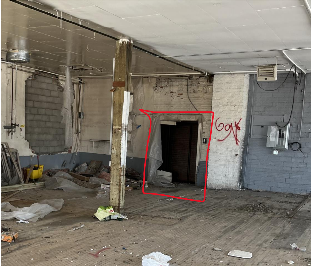
Second floor, red box indicates open elevator shaft.
