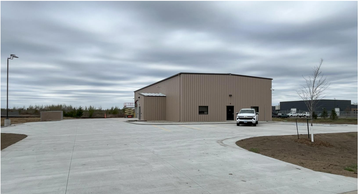
Finishing touches still being added to the Border States new building in the Technology Park, October 9, 2025
