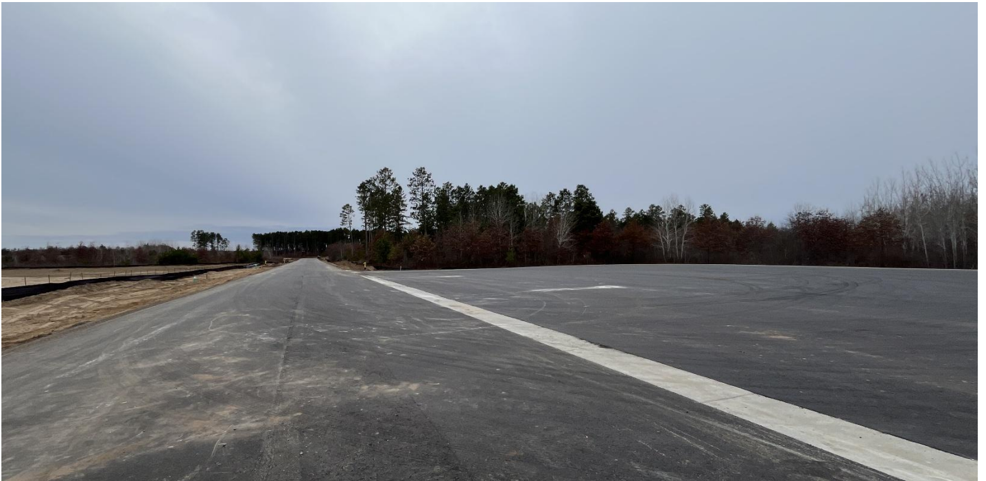
Road paving complete and landscape stabilization in progress at Bemidji Airport Planning Area 3, November 4, 2025
