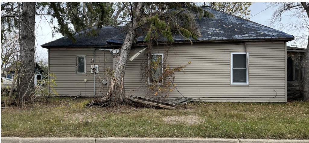
Property with unresolved storm damage.
