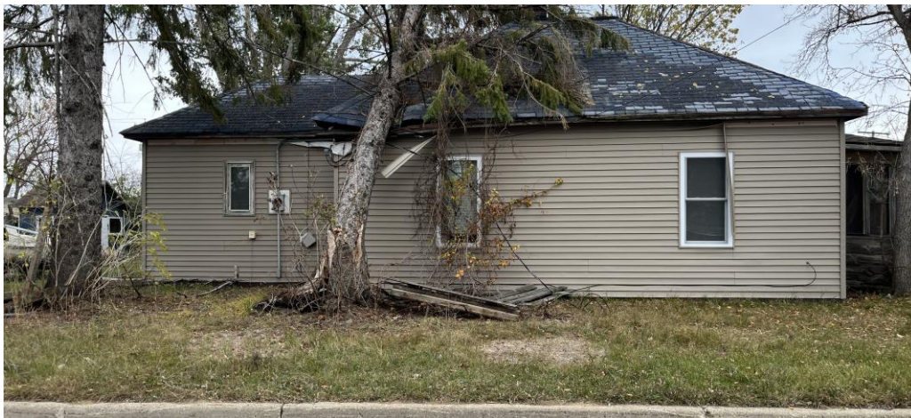
Property with unresolved storm damage.
