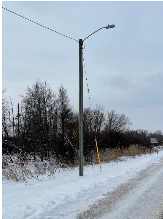
Typical wooden pole with pole mounted mast arm with LED light
