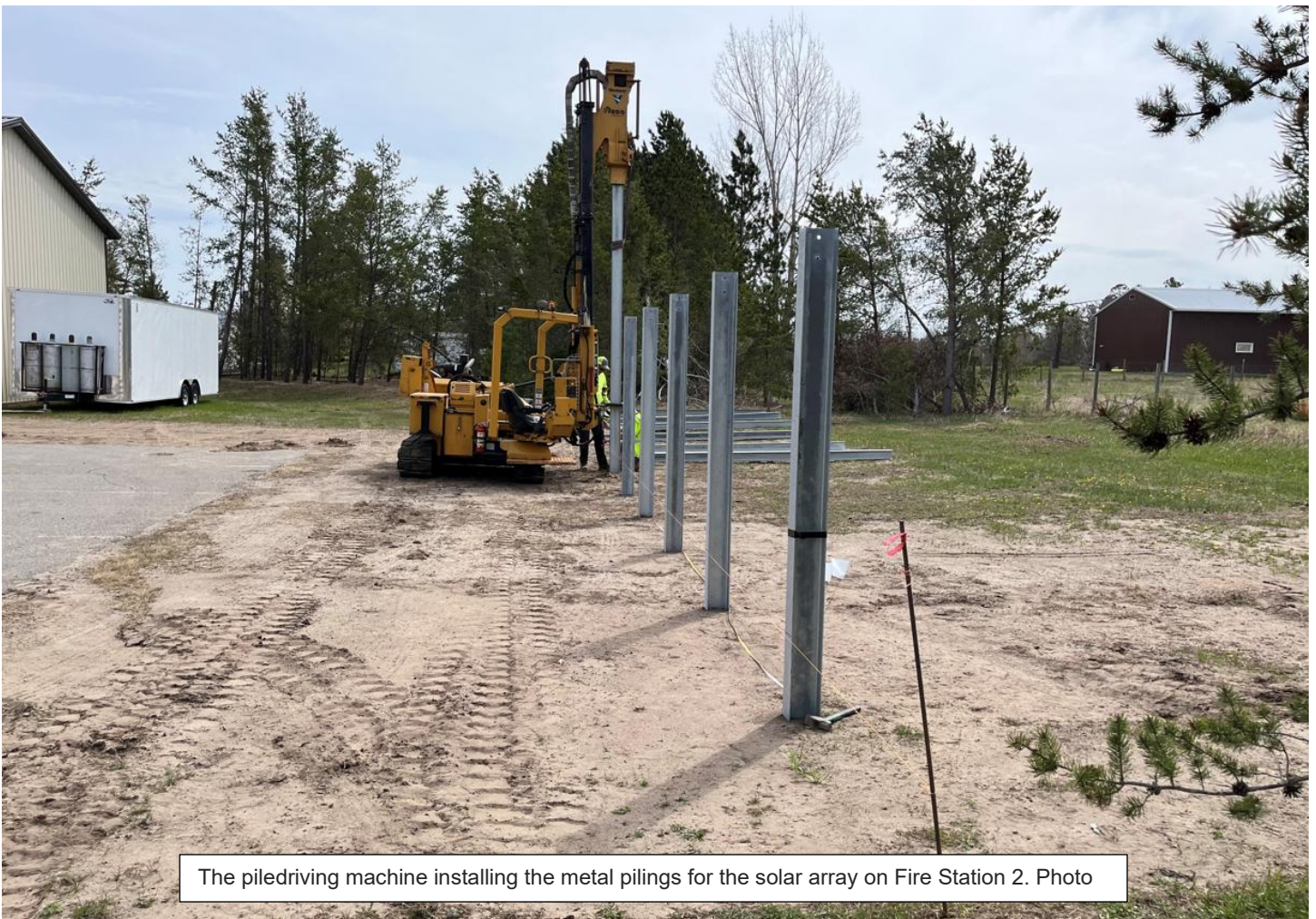
The pile-driving machine installing the metal pilings for the solar array on Fire Station 2. Photo
