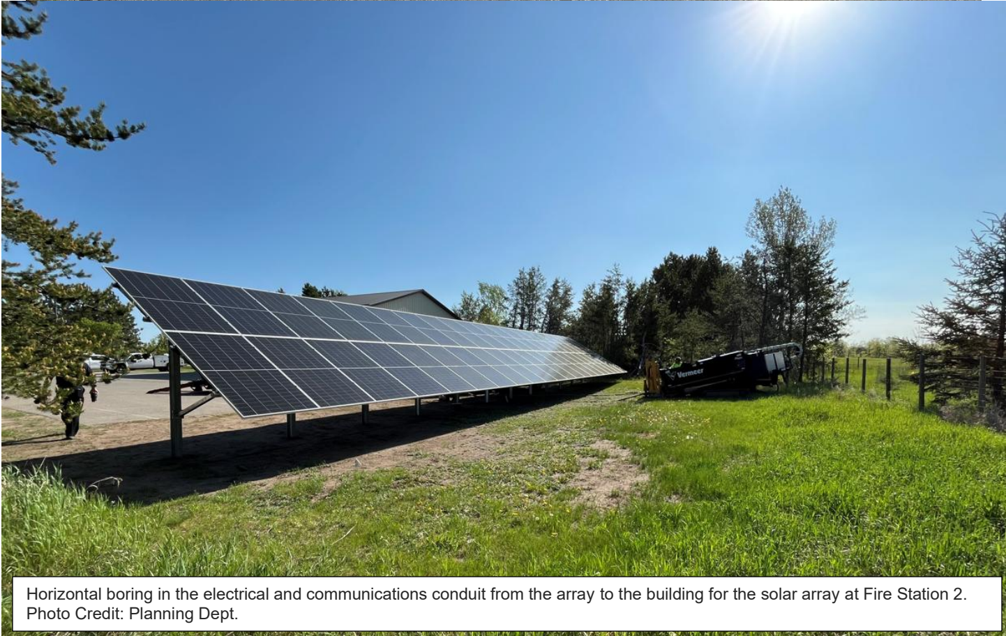
Crews getting set up to start work for the solar array at Fire Station 2. Photo Credit: Planning
