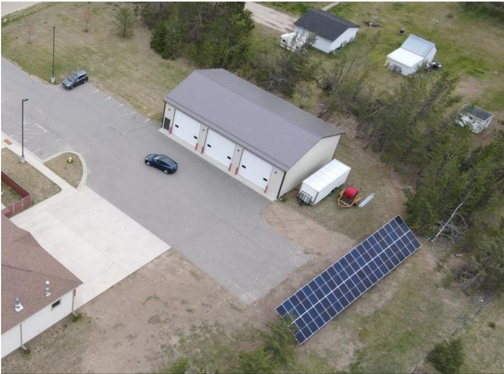
Drone shot of the newly installed solar array on Fire Station 2. Photo Credit: Planning Dept.
