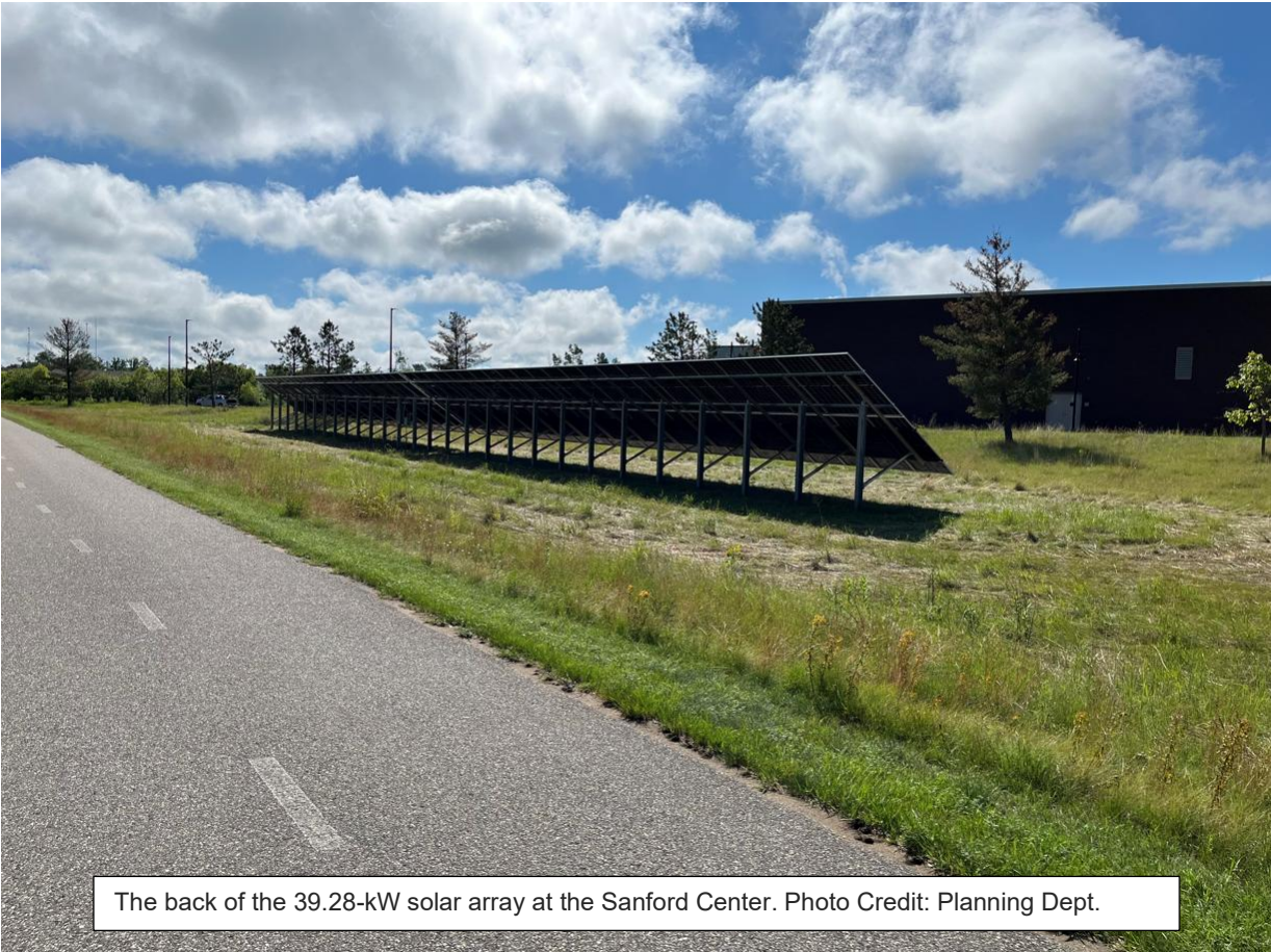
Sanford Center 39.28-kW solar array looking northeast. Photo Credit: Planning Dept.
